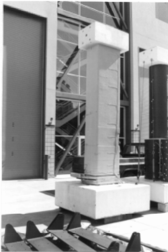
Fig. 2: Rectangular Column Retrofitted Using Carbon/Epoxy Tow Preg and Subsequently Covered With a Protective Coating
