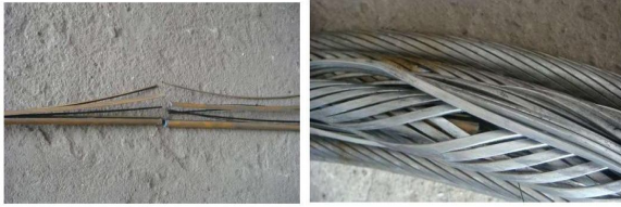
Fig. 9. In service failures of ACCC conductors [18].
