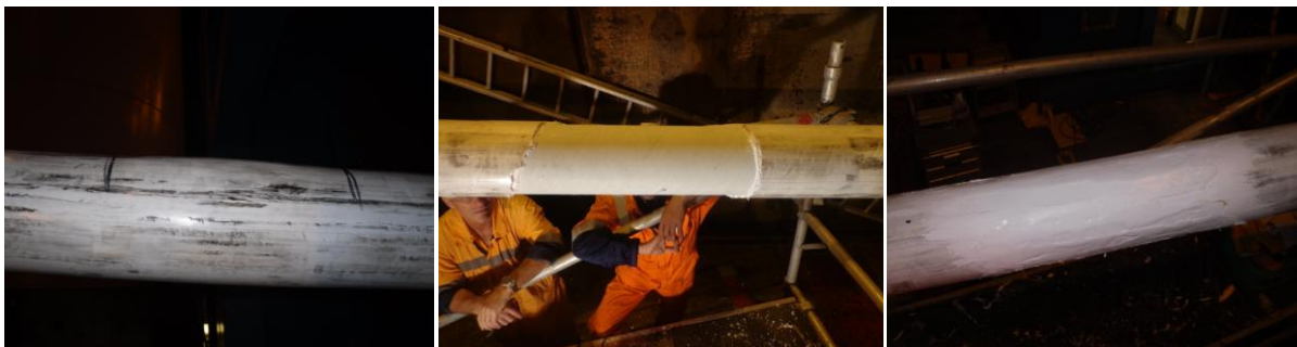
Figure 6: Coating repair after tensioner malfunction
